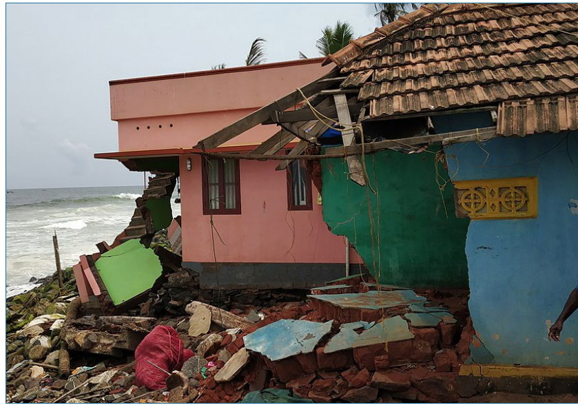
Figure 1. Coastal erosion destroys houses at Valiyathura, Kerala, India
